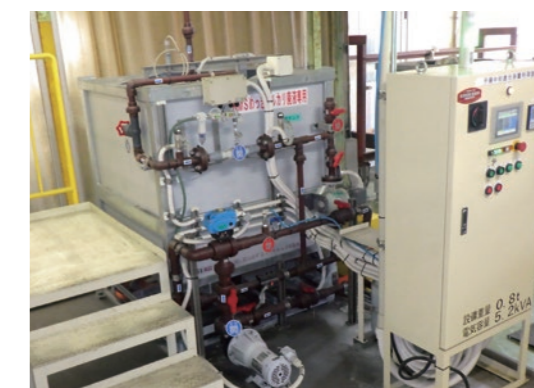
Wastewater treatment equipment
