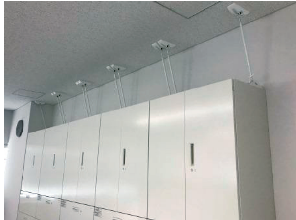
Photo 6 Product installed at KYB Kumagaya Plant for monitoring purpose
