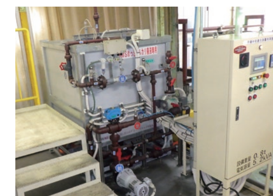
Wastewater treatment equipment
